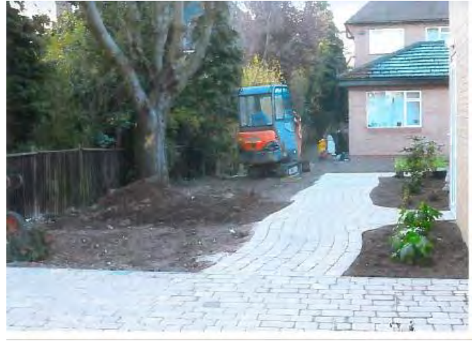
Physical damage and Tree removal
